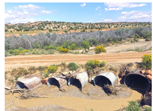
Alvey Wash. Large culverts fill with sediment during storm events.
