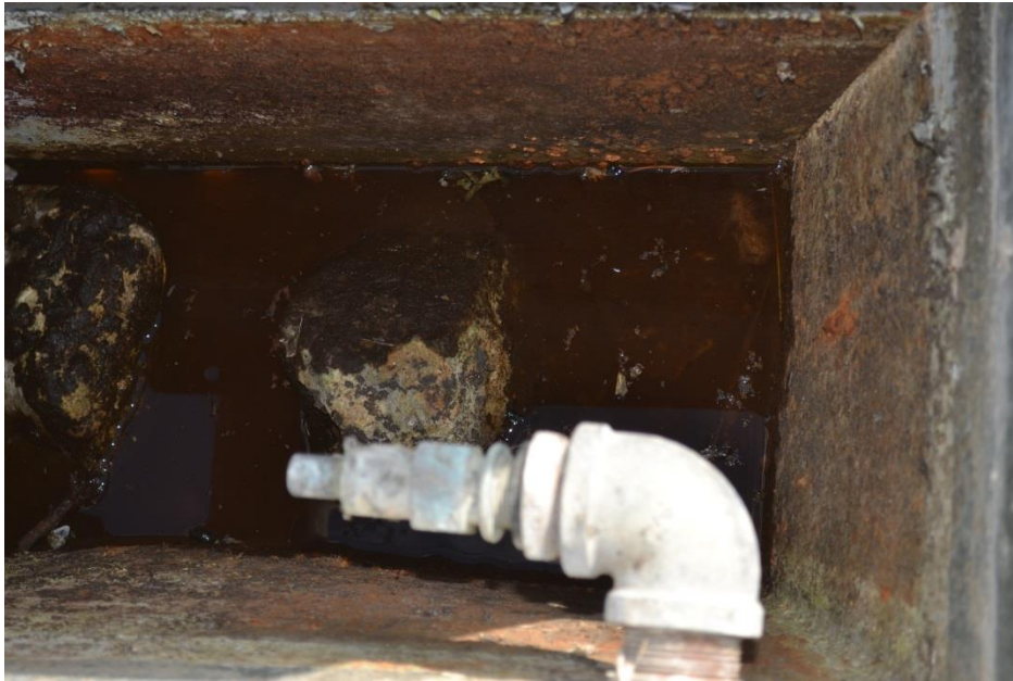
Figure 28. Summit spring October 2016. No water flowing from from spring. Outlet from spring pictured above with no water flowing from pipe.
