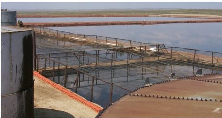
Oilfield wastewater disposal facility. USFWS/Pedro Ramirez, Jr.
