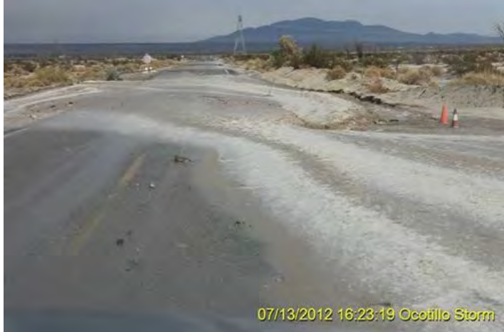
Unknown leftover foam from a chemical dust suppressant was spread everywhere when the Ocotillo Wind Express project site flooded in June, 2012
