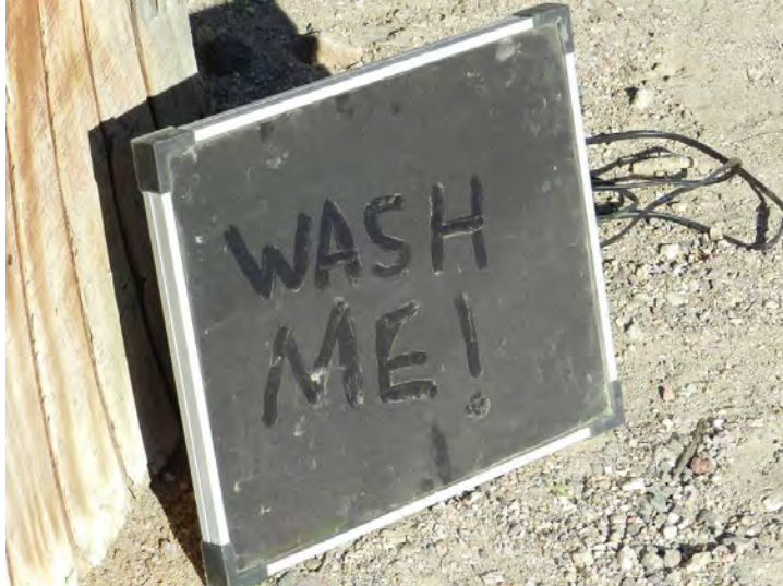
^Dusty photovoltaic panel
