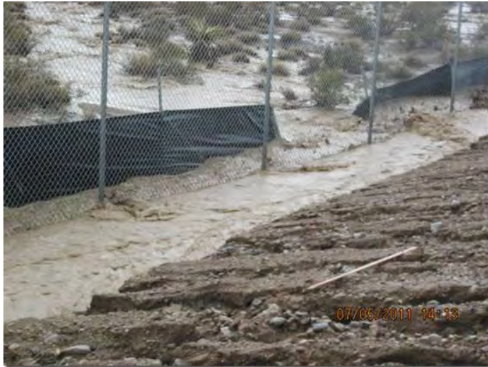
^Ivanpah Solar Electric Generating System: desert tortoise exclusion fence removed by floods. July, 2011
