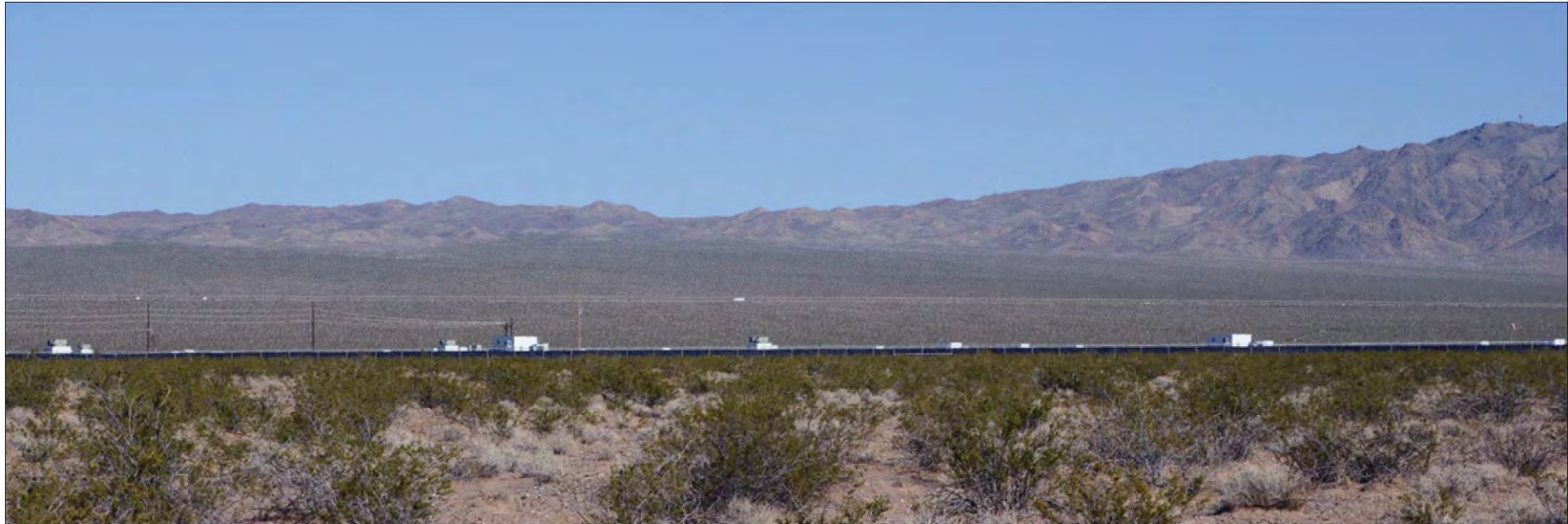
Inverters Painted White
