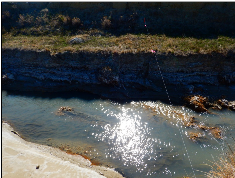
PHOTO 2.22. SITE A3 LOOKING AT LEFT BANK OF CROSS SECTION 1 NOTE SHEAR BLOCK FAILURE
