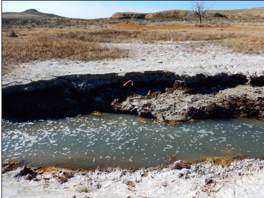
PHOTO 2.25. SITE A3 LOOKING AT LEFT BANK OF CROSS SECTION 6 NOTE SHEAR BLOCK FAILURE/SLOUGHING
