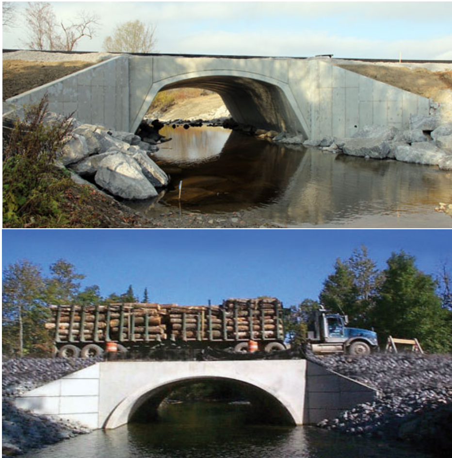
Figure 4. Example Perennial Stream Crossing Pre-Cast Concrete Arches
