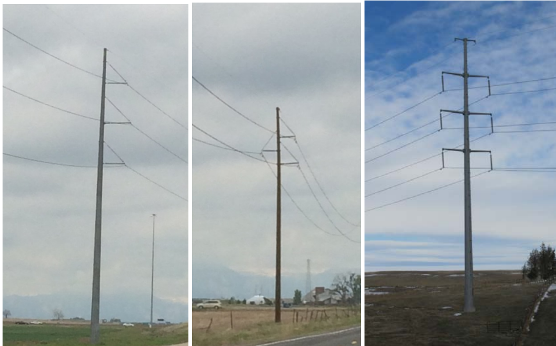
Figure 4-21. Typical Monopole Transmission Towers
