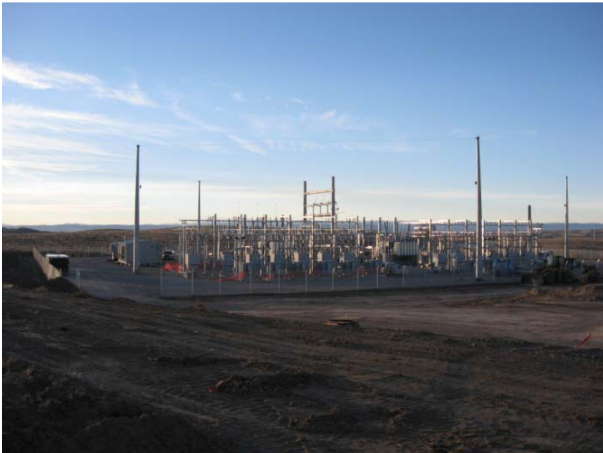
Figure 4-20. Example Wind Energy Collection Substation
