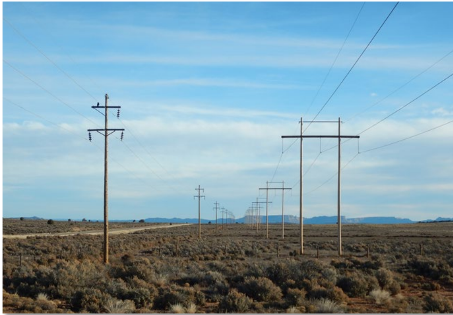
Examples of a 69kV single wood pole (left) and 138kV H-frame (right) in Grand Staircase-Escalante National Monument
