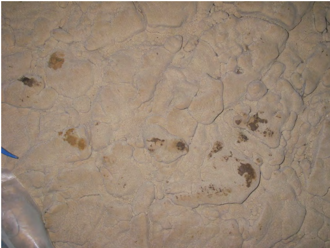
Before and after (the wet spots will dry). – note broken “Easter egg” on right of photo below which cannot be repaired. In many areas the staining on the calcite can’t be removed.
