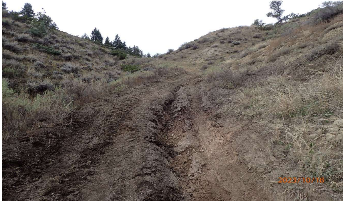
Figure 2. Example of severe erosion within the traveled way (47.891363, -109.018562).
