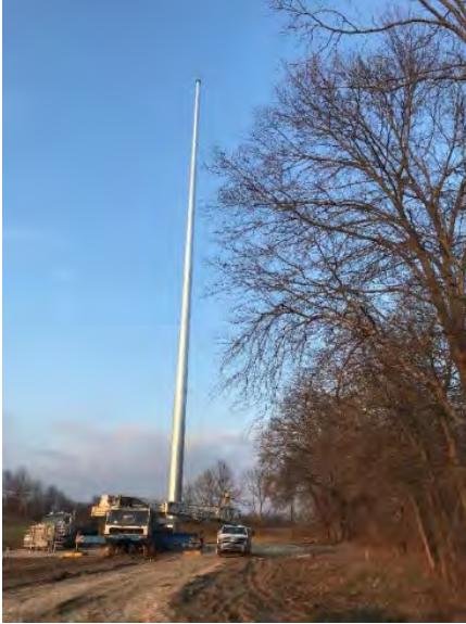
Figure 1-9. Typical Monopole Met Tower
