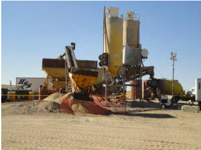
Figure 1-12. Typical Temporary Concrete Batch Plant
