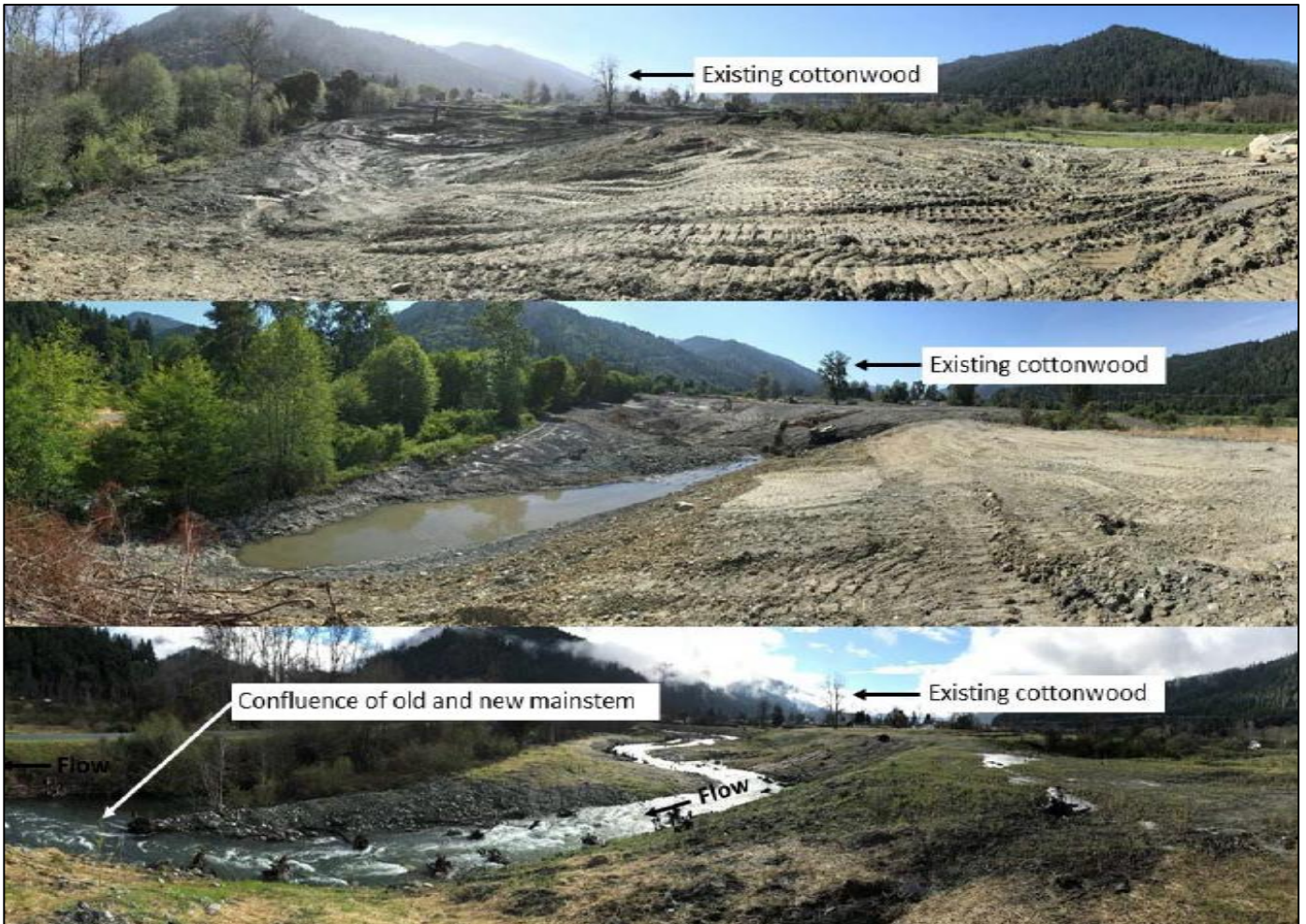
Figure 3. Watershed restoration activities at Mill Creek, during construction (top and middle) and after construction (bottom).
