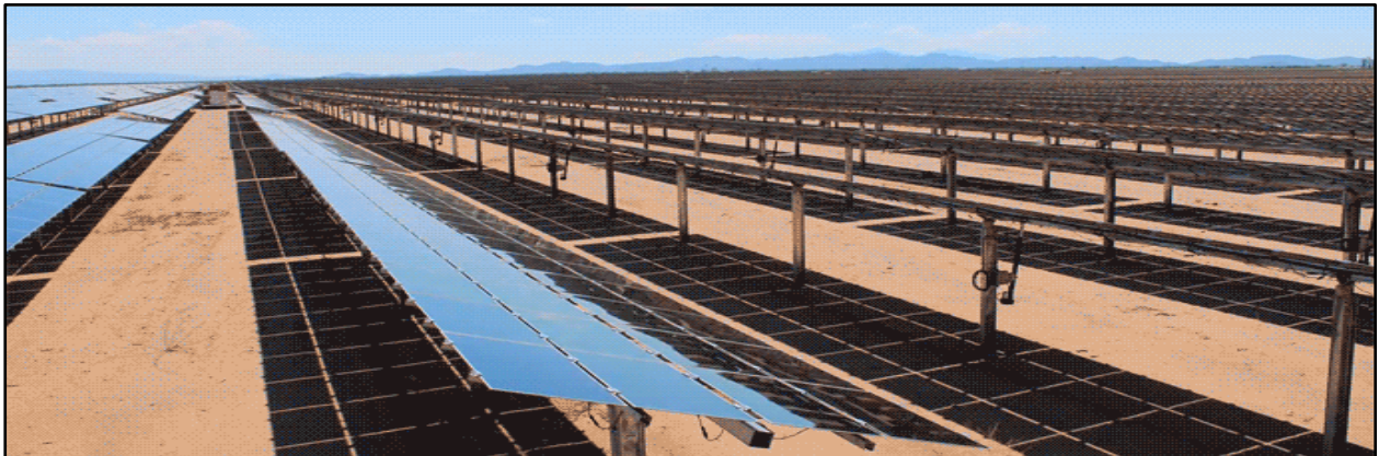
Figure 2-4. Typical PV Module Tracking Structure
