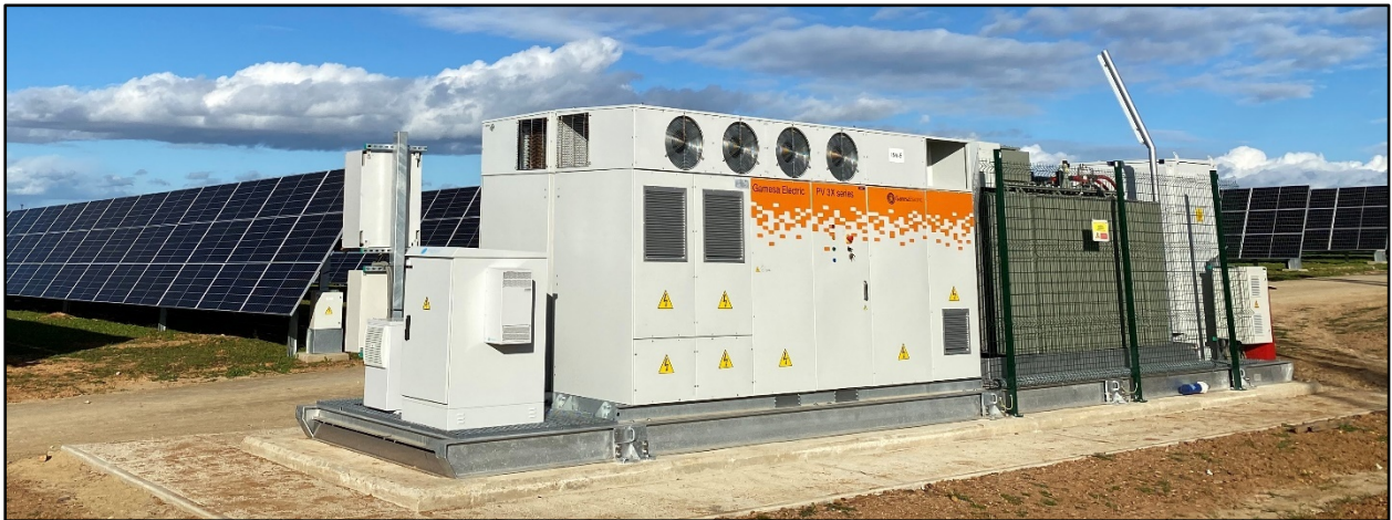
Figure 2-5. Typical Inverter Station
