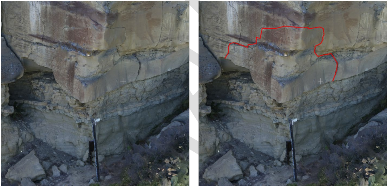
Figure 22 Signature Block 2 rock breakage.
