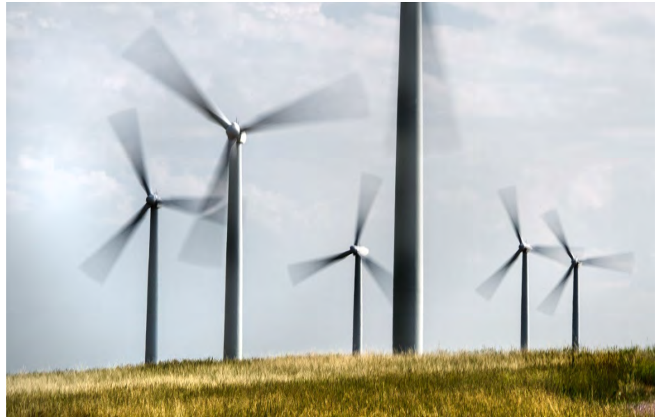
Combination of 221 Mitsubishi Heavy Industries 1-MW turbines and 53 GE 1.5-MW turbines at the Cedar Creek Wind Farm in Grover, Colorado. Photo by Dennis Schroeder, NREL 30593
