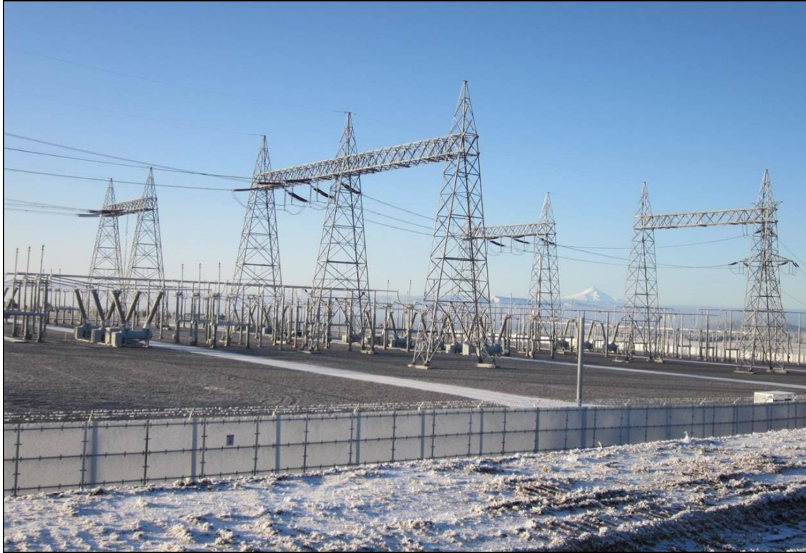
Figure A3-6. Typical 500-kV Station
